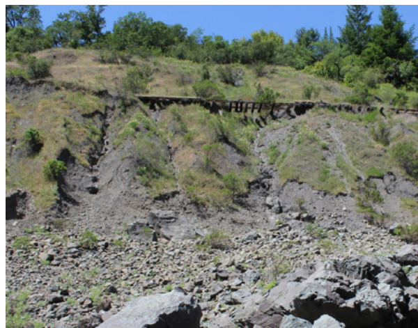
Eroded railway embankment in Eel River Canyon
