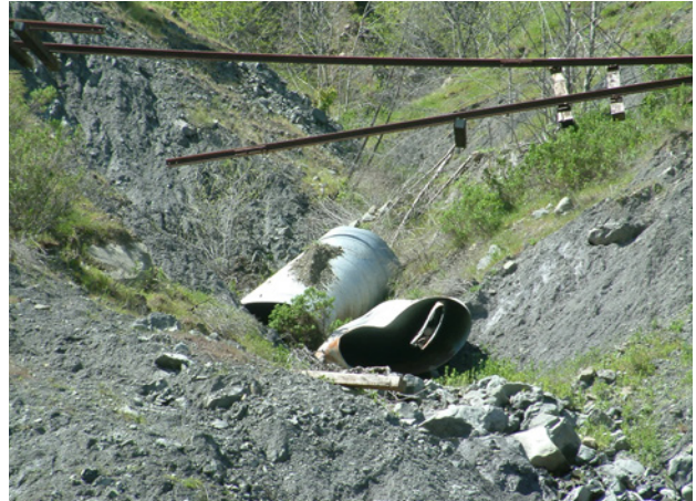
Existing failed culvert
