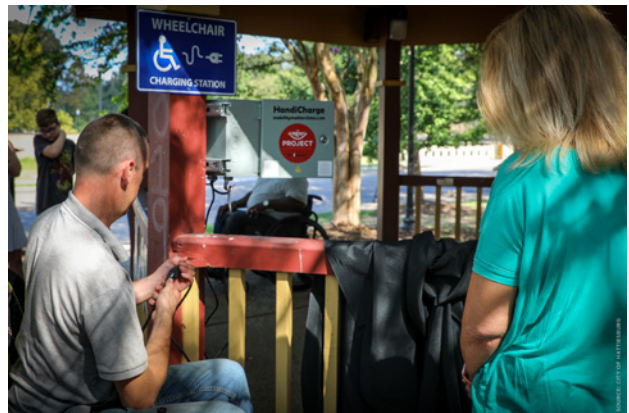
The City of Hattiesburg, Mississippi has installed nine publicly accessible wheelchair charging stations
