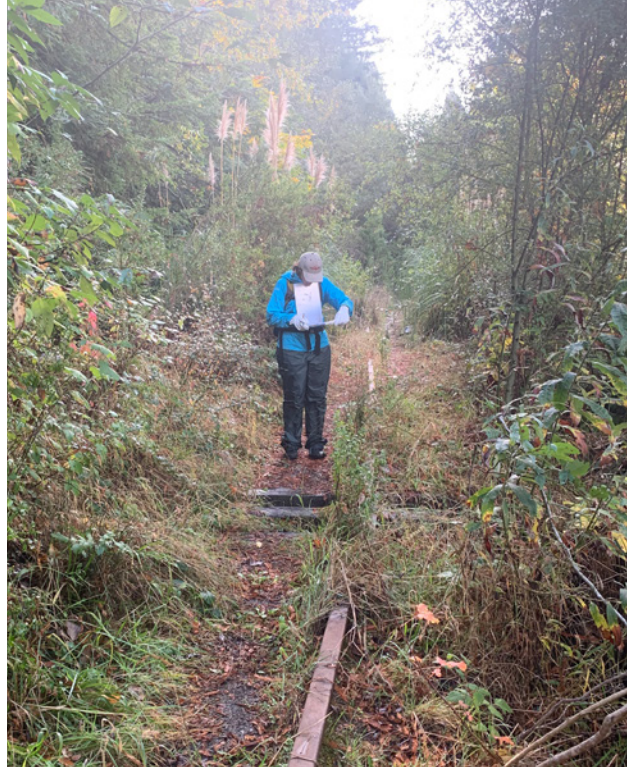
Existing culvert failure
