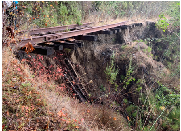
Existing failed culvert
