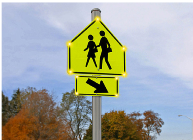
Flashing beacon with push button
