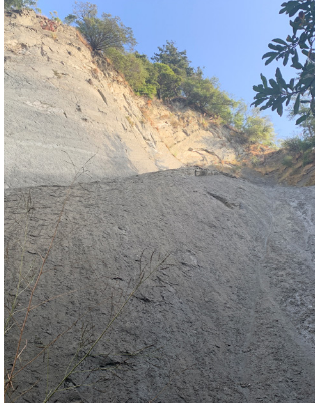
Landslide and steep slope along corridor
