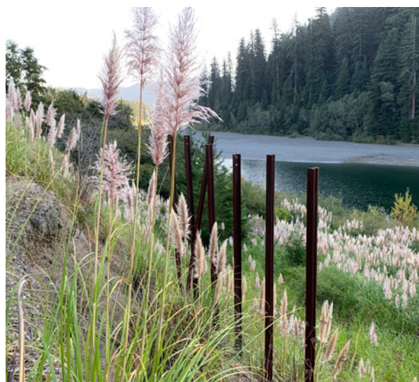
Failed wall along the Eel River
